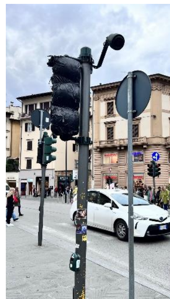
Ineffective bagging of a signal head
