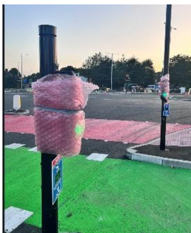
bubble wrap covering active wait box
