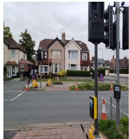
wait boxes not bagged and close together. Siting of portable pedestrian signal not effective.
