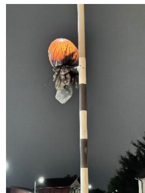
plastic cover showing light on beacon
